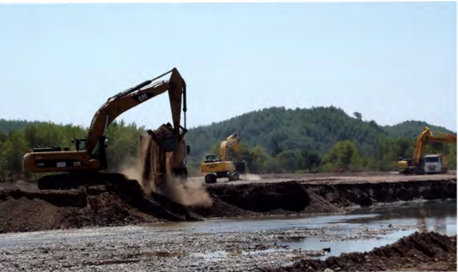
Views from Antalya Aksu River flood protection
