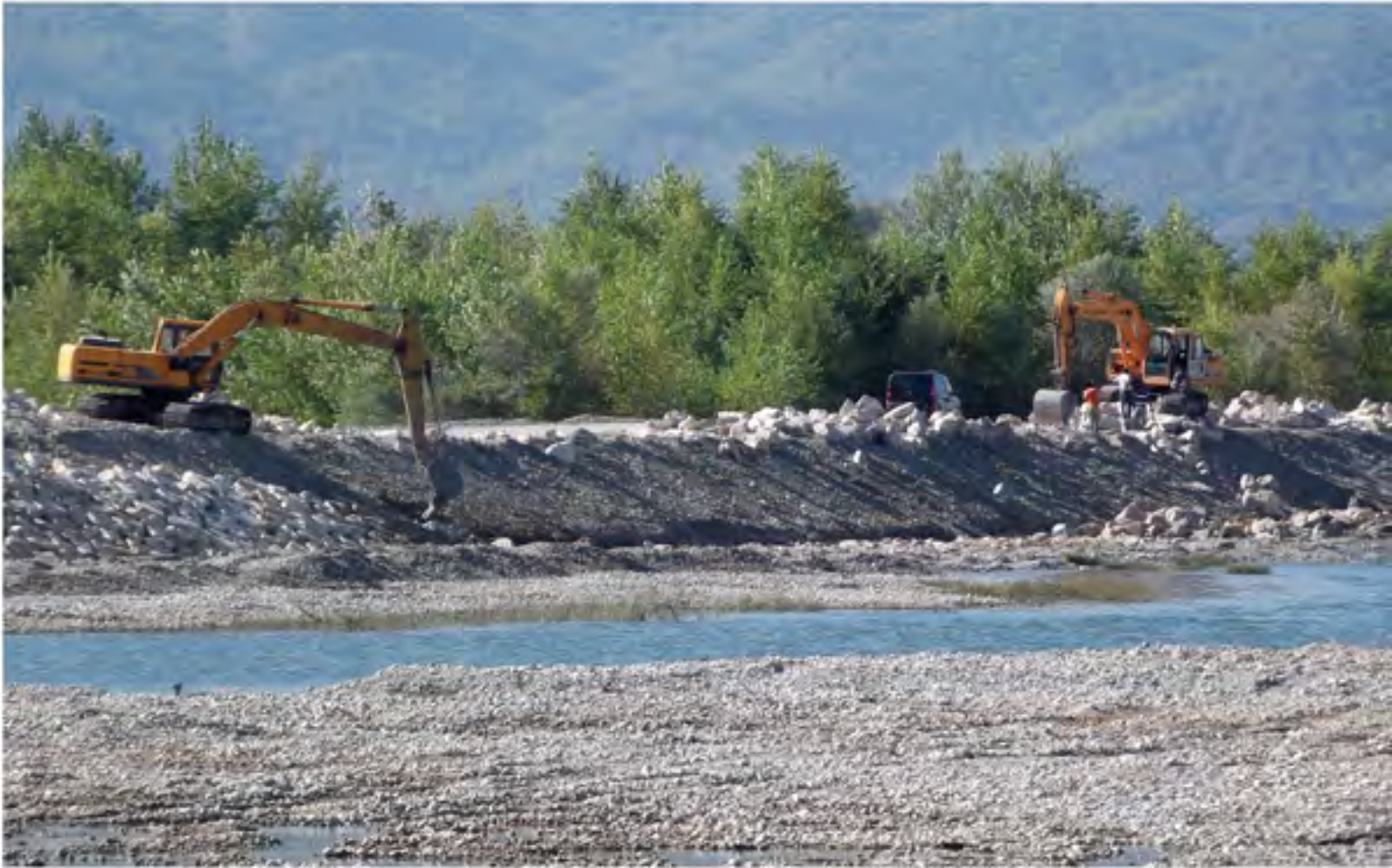
Views from Antalya Aksu River flood protection
