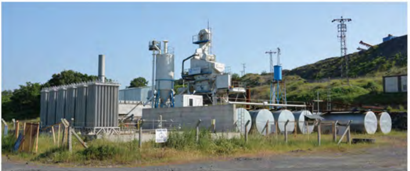
Asphalt Batching Plant facilities
